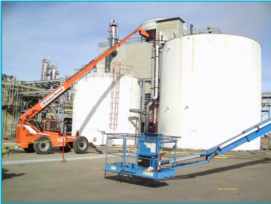
Photo left: East neutralization tank
