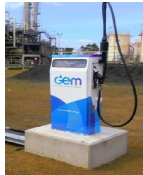
Methanol / gasoline pump at Coogee plant site
