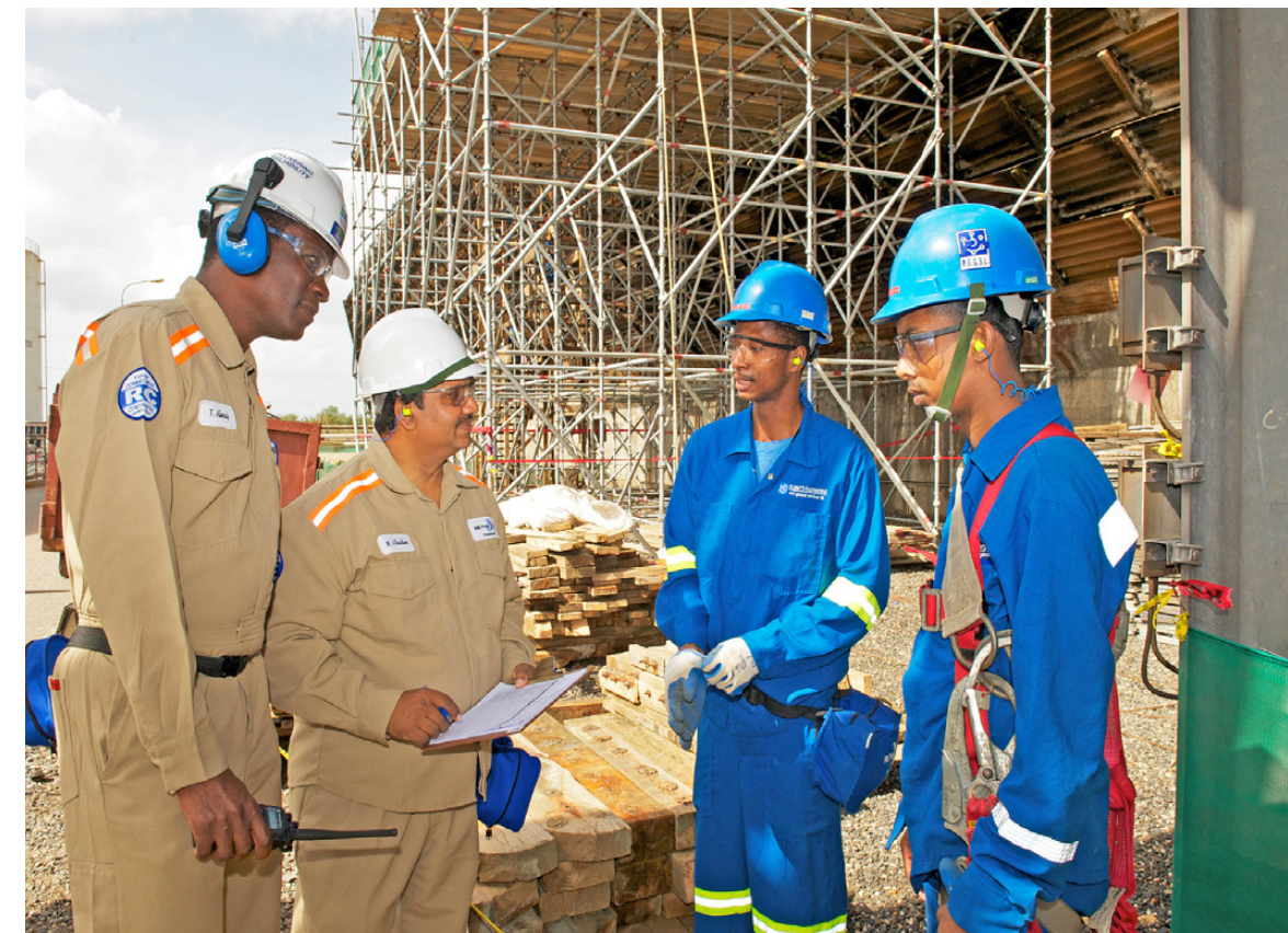
Rudy Chadee, Director, Finance (2nd from left) was accompanied by Theron Alexis, Manager, Maintenance (left), for a safety audit of a job on the Atlas Cooling Tower, interacting with contract workers Rodney Pierre (2nd from right) and Visham Lochan.
